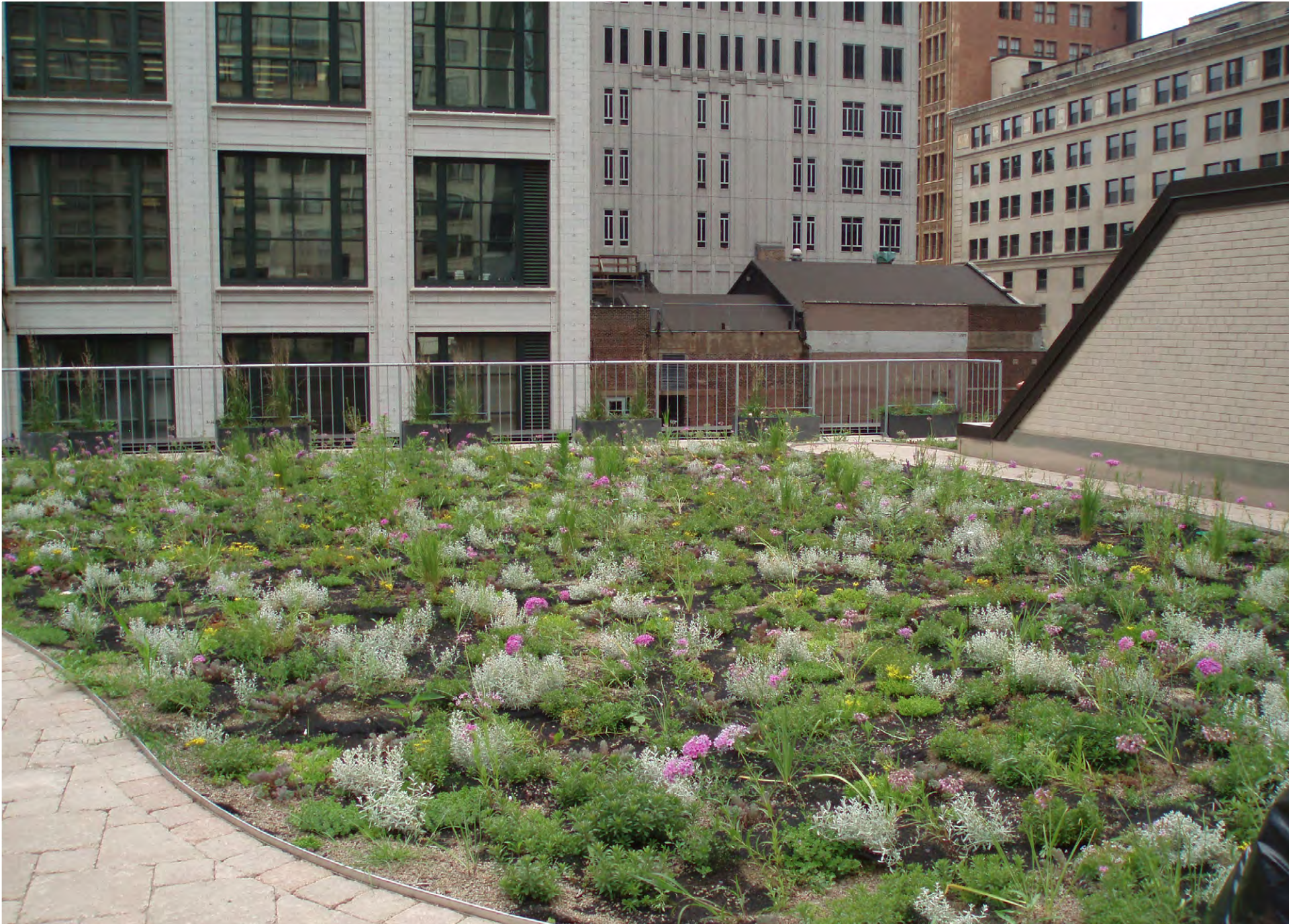
GSA Region 5 - 10 West Jackson Street Building, Chicago, Illinois A 12,000 square foot extensive green roof replacement of an existing, modified bitumen (black) roof.
