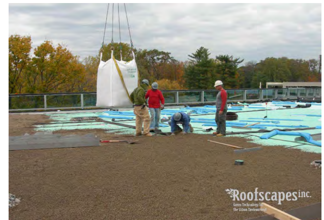
Use of protective equipment such as hard hats and steel-toed boots during green roof installation
