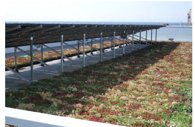
Photovoltaics installed on the United States Environmental Protection Agency Region 8 Headquarters, Denver, Colorado
