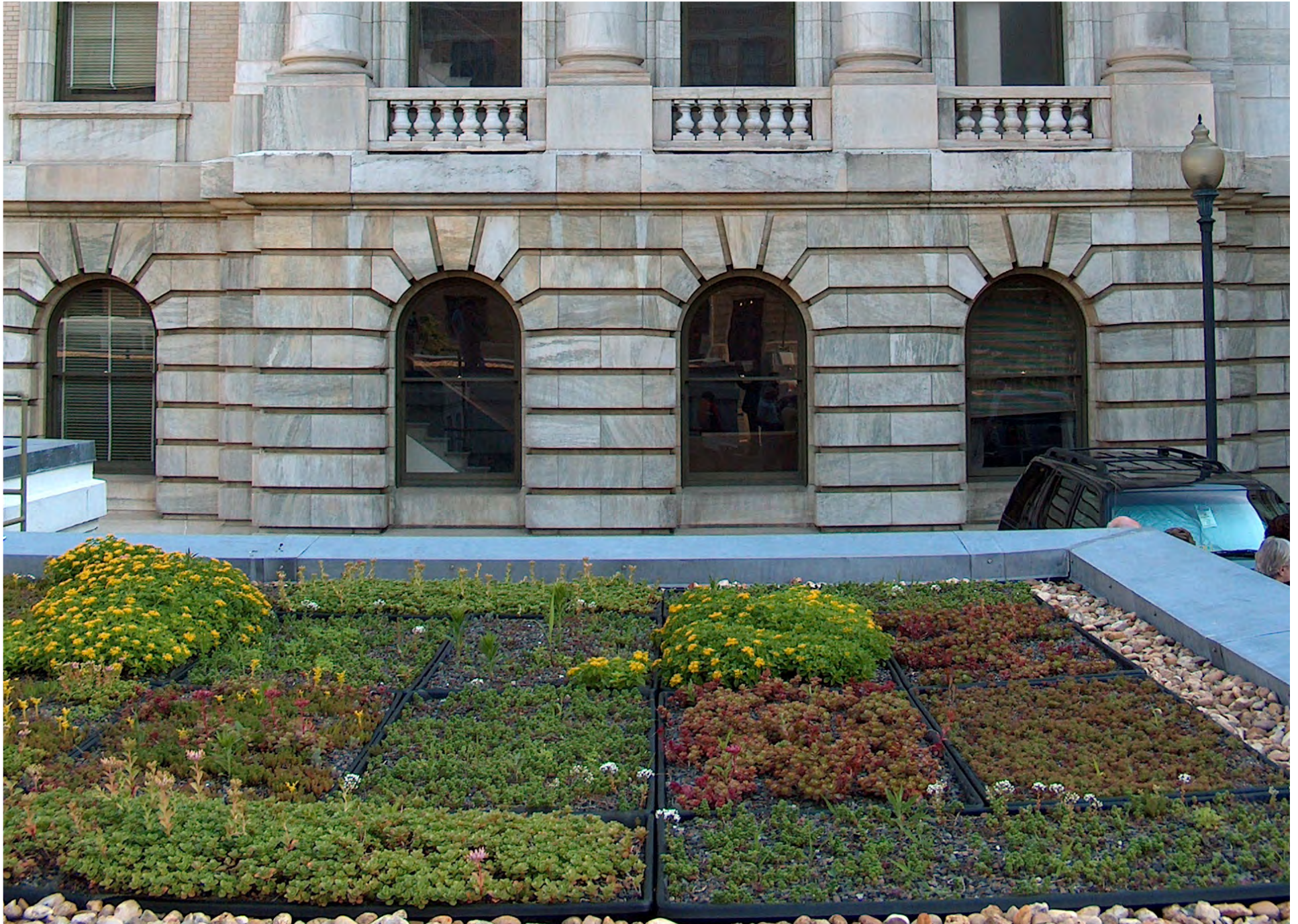
GSA National Capital Region - United States Department of Agriculture Jamie L. Whitten Building, Washington DC A 3,700 square foot modular, extensive and accessible (via pedestrian path) green roof installed on this historic building that projects into the National Mall.
