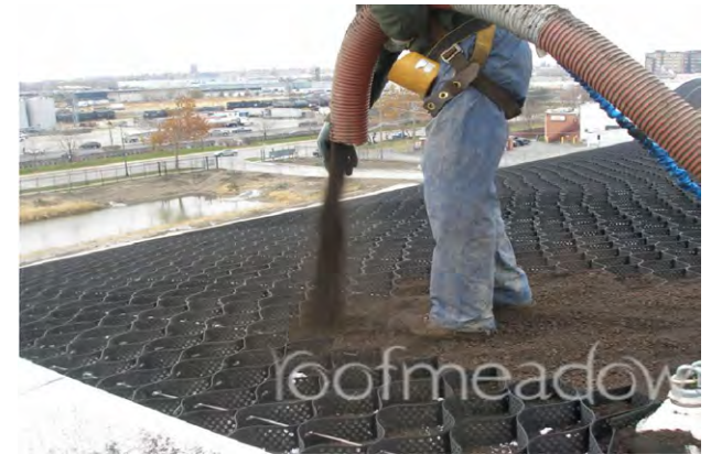
Green roof contractors using a pneumatic blower to install the growing medium
