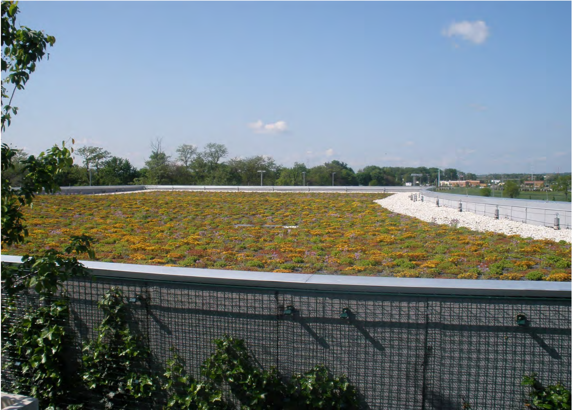
GSA Region 3 - FEMA Disaster Operations Center, Winchester, Virginia A 50,000 square foot extensive green roof planted on the new LEED Certified building (2008).
